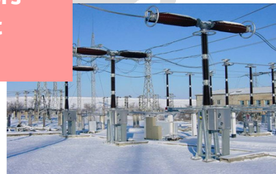
Air Insulated Substations
