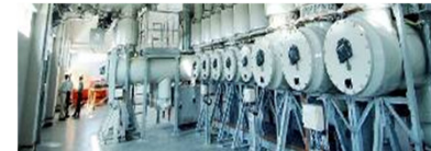
Next generation substation
