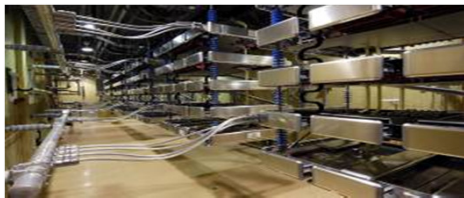
High Voltage Direct Current
