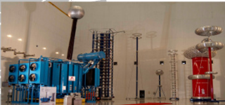
Vadodara, India Power Transformers factory
