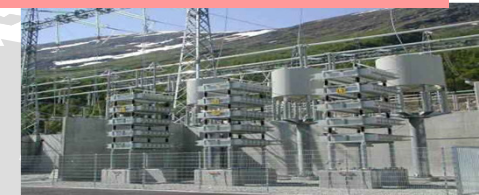
Flexible Alternative Current Transmission Systems Special Solutions for industries
